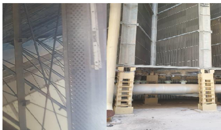
Figure 2. View of a delta unit and the arrangement of tubes in the dry tower
